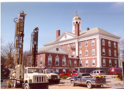
City Hall – Geothermal System
